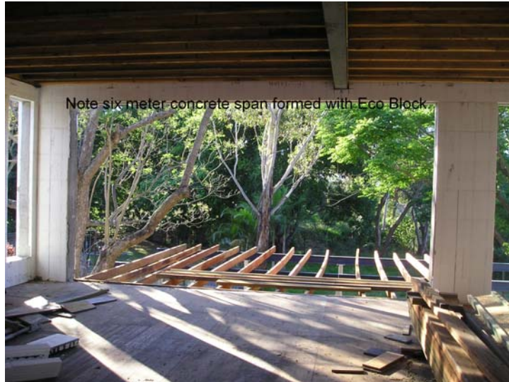
(7) Lintels over door and window openings are formed using Eco Block and rebar to provide additional strength. Please refer to our engineering tables for further details.
