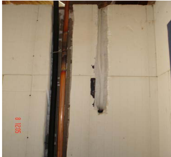
(5) Example of electrical installation
