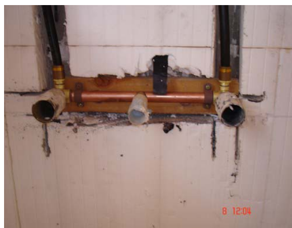
(4) Example of plumbing installation
