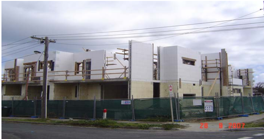
(9) Apartments being built by Andrew Polydorou (Eco Block builder & Distributor) in Victoria
