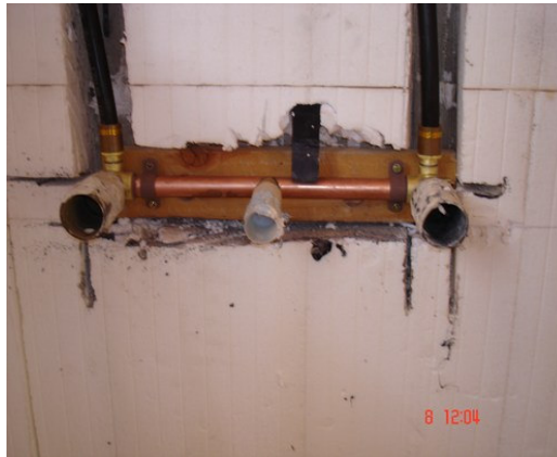
Example of plumbing installation
