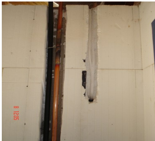
Example of electrical installation & plumbing
